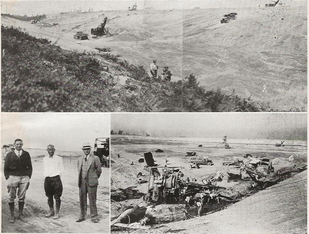
In the upper photograph is shown sizeable hill that had to be removed before Seattle's 75,000,000-gallon water reservoir could be constructed. Lower left, from left to right: W. H. Stillman, special sales representative of the Union Oil Company in Seattle, R. S. Seabrook and C. M. Elliott of the contracting firm, Elliott, Stroud Bros. & Seabrook, excavation contractors on the project. Lower right, the reservoir as it appeared with the excavation work virtually completed.
