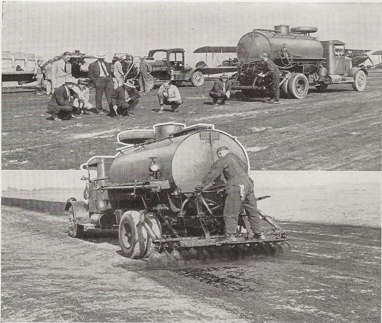
In the top photograph you see representatives of the American Aircraft Company, Ltd., and the Union Oil Company inspecting one of the airport's 3000-foot taxi lanes, which a few minutes later was sprayed with Union road oil, as is shown below.
