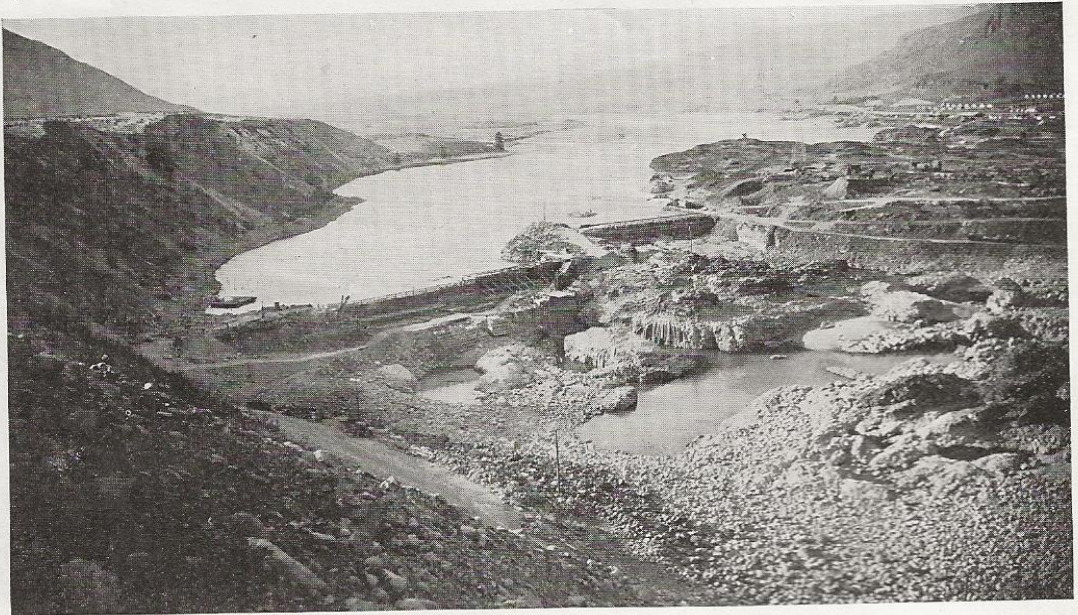
A view of the upper cofferdam at Rock Island where the Stone & Webster Corporation is building a $19,000,000.00 dam across the Columbia River. On the right is shown the northern end of Rock Island and in the foreground the nearly dry bed of the Columbia River between the two cofferdams. Water is being pumped out as rapidly as possible so that work on the actual construction of the dam may begin.
