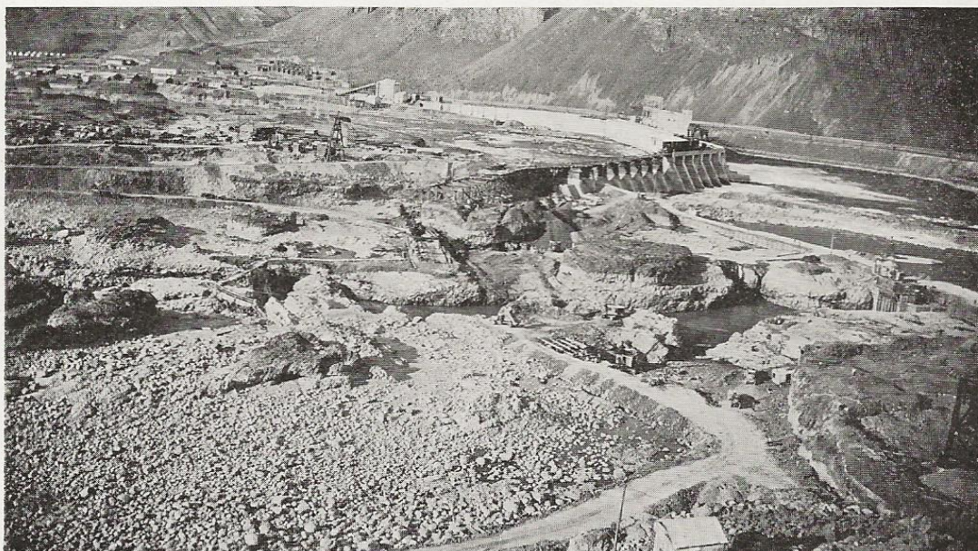
The completed portion of the dam across the East Channel of the Columbia River appears in the distance in this photograph. In the foreground and to the right can be seen the lower cofferdam holding back the waters of the river from the stream bed of the West Channel.
