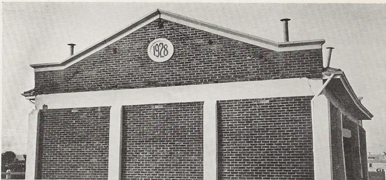
The above photograph shows how Hastings' case goods plant looked just after earthquake struck. Note cracks all through the building.
