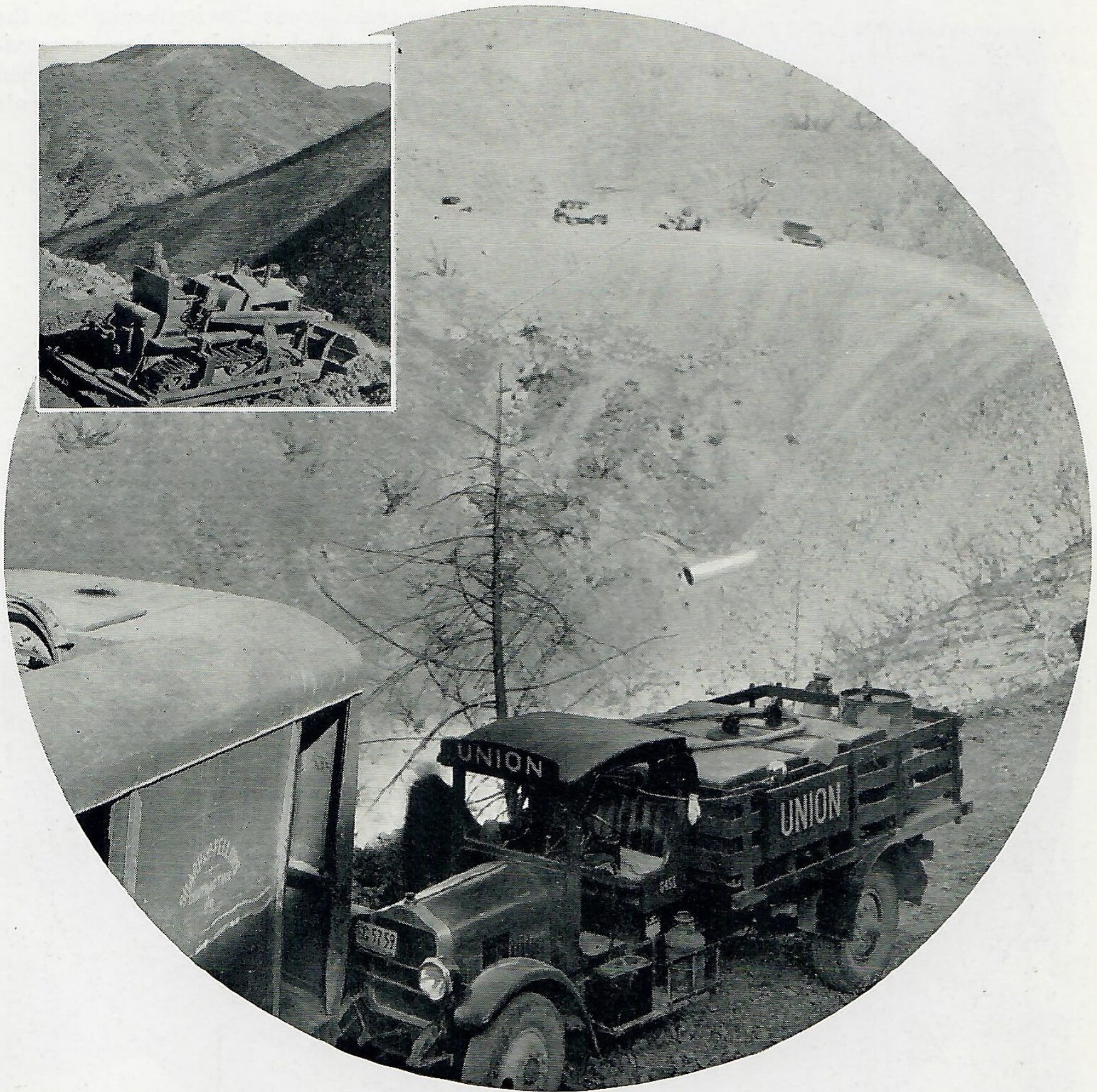
Lima "101" shovel receiving gasoline during halt in grading operations on Maricopa-Ventura shortcut over Sespe mountains, and above, inset, showing tractor equipped with bulldozer in action.
