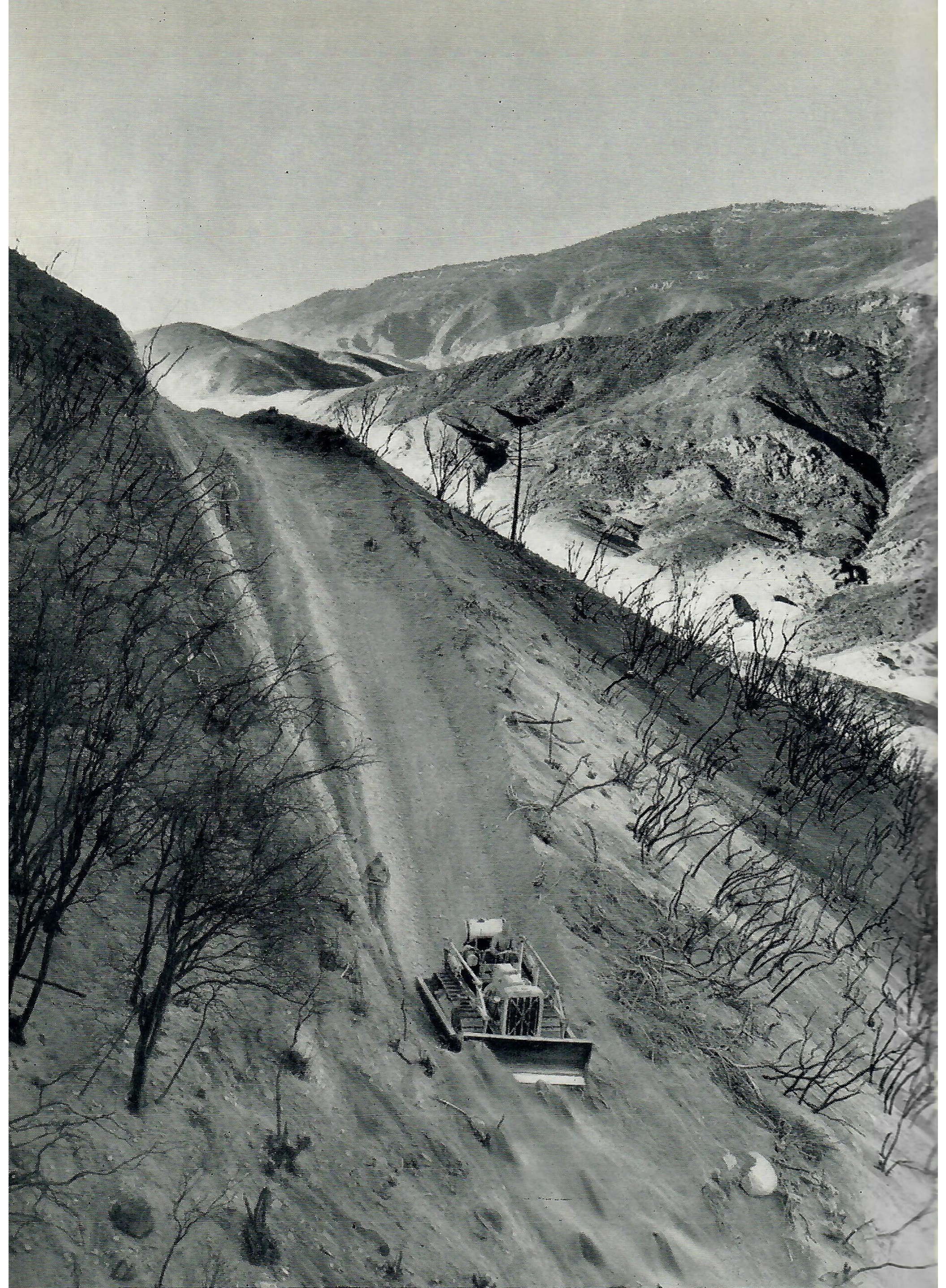
This Diesel-powered tractor, equipped with bulldozer, is carving the way for the new Maricopa-Ventura shortcut through the Sespe mountains. A tractor-drawn sled is used to haul fuel over the mountain ridges to the tractor.
