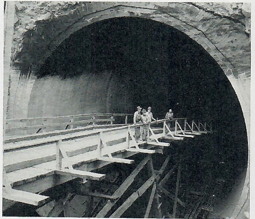
Completed end of diversion tunnel No. 3. Elevated roadway carries concrete and muck trucks back to other end of tunnel. Size of the circular bore, through which waters of Colorado will run during construction of dam proper, can be appreciated when compared to the men standing on the runway.
