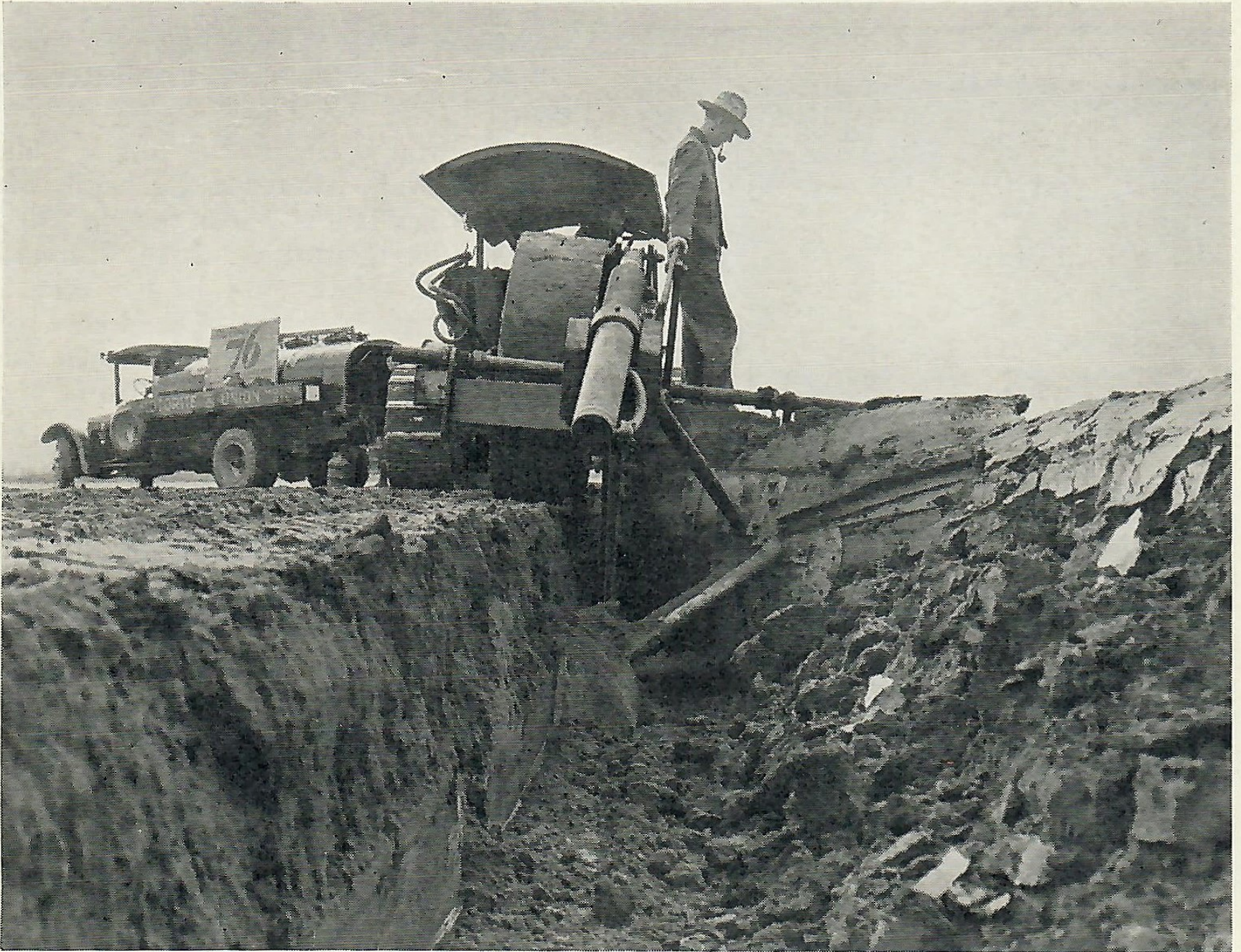
The 36-inch trench which the Plaven plow upturns is shown in this photograph. The three tractors required to pull the plow had just been fueled with new Union 76 gasoline when this picture was taken. For the past seven years Paul Plaven, builder of the plow, has been a consistent user of Union Oil Company products.
