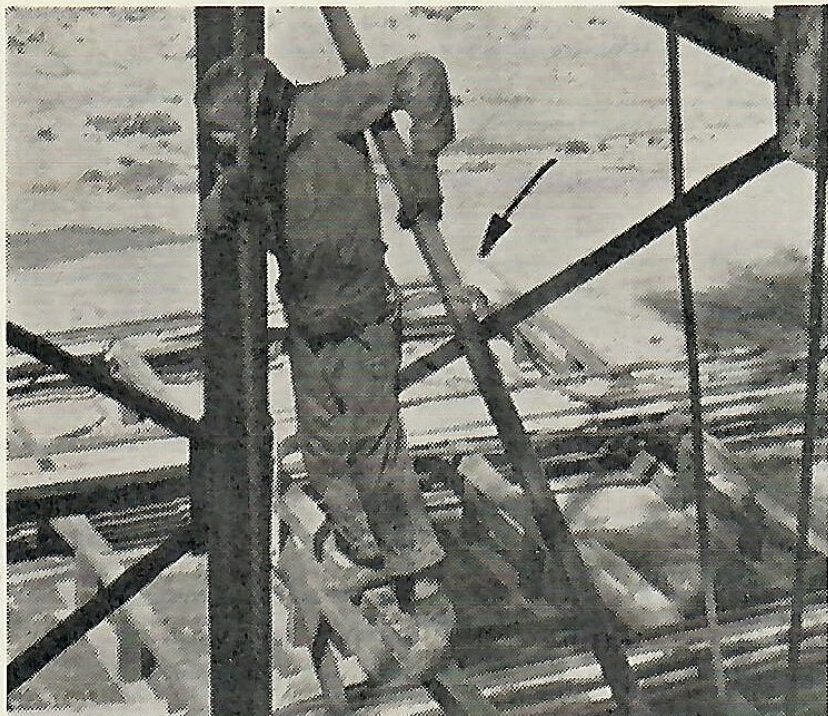
If stops have to be made in the derrick, the little line is snapped around a girt or brace.
