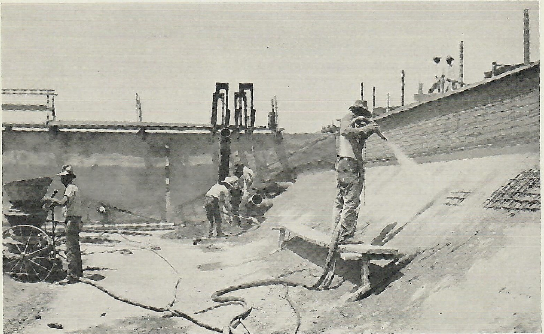
This picture indicates the method of applying concrete on the walls and floor of the separating reservoir. The concrete is shot on under heavy air pressure through a nozzle, becoming very dense and hard. At the left is the mixing chamber or carburetor where proper proportions of sand and cement are introduced.
