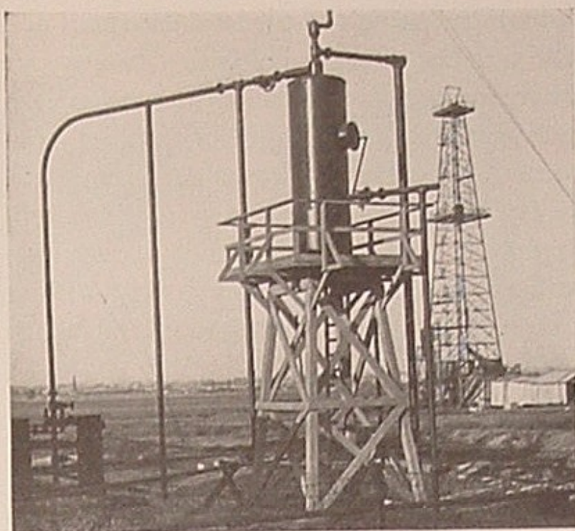
The gas trap, which collects the natural gas from the main body of oil
