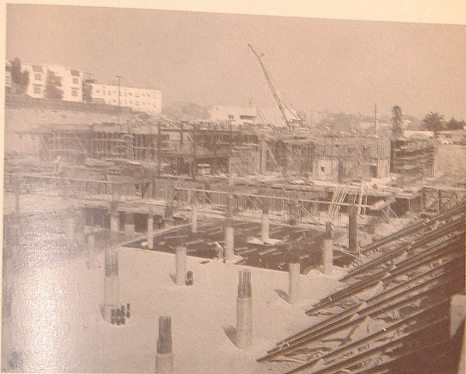
August 1956: Workmen are about ready to pour concrete for the ground floor or lobby level of the 13-story Home Office Building. From this level steel columns and girders will soon rise to give the project full definition. In the parking area, pillars continue to grow; concrete has just been poured for the ramp (left center) leading down to D level.
