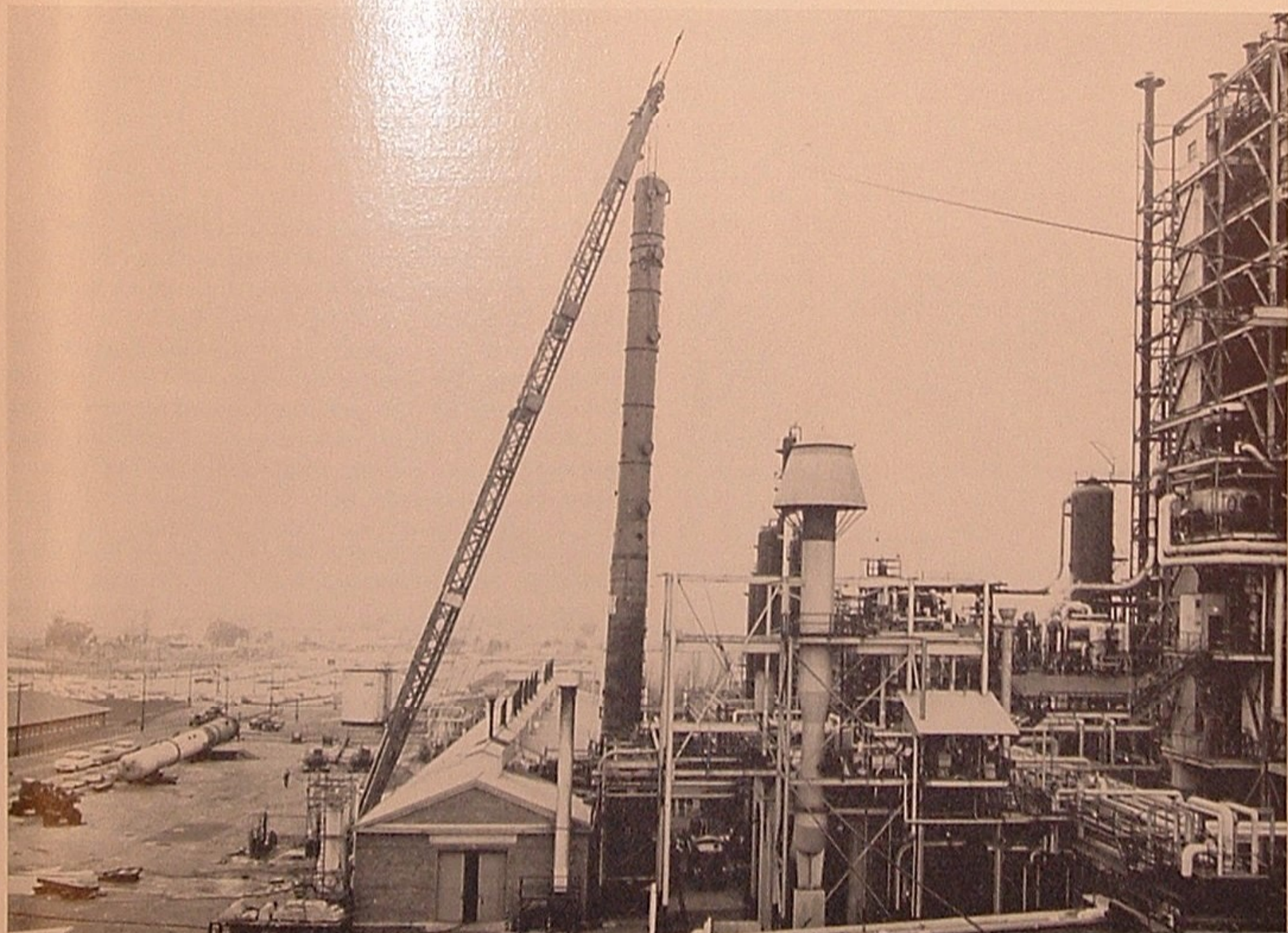
In position to be bolted down for many years of service is the new De-ethanizer. The job was achieved according to plan and without evidence of backstrain.
