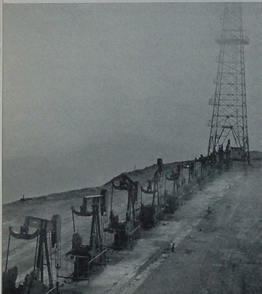
"CARAVAN" is the impression given by this string of pumping units in our South Mountain Field near Santa Paula. They are actually faced with an up-hill climb in helping satisfy the crude oil needs of California. Photo by Will Connell.
