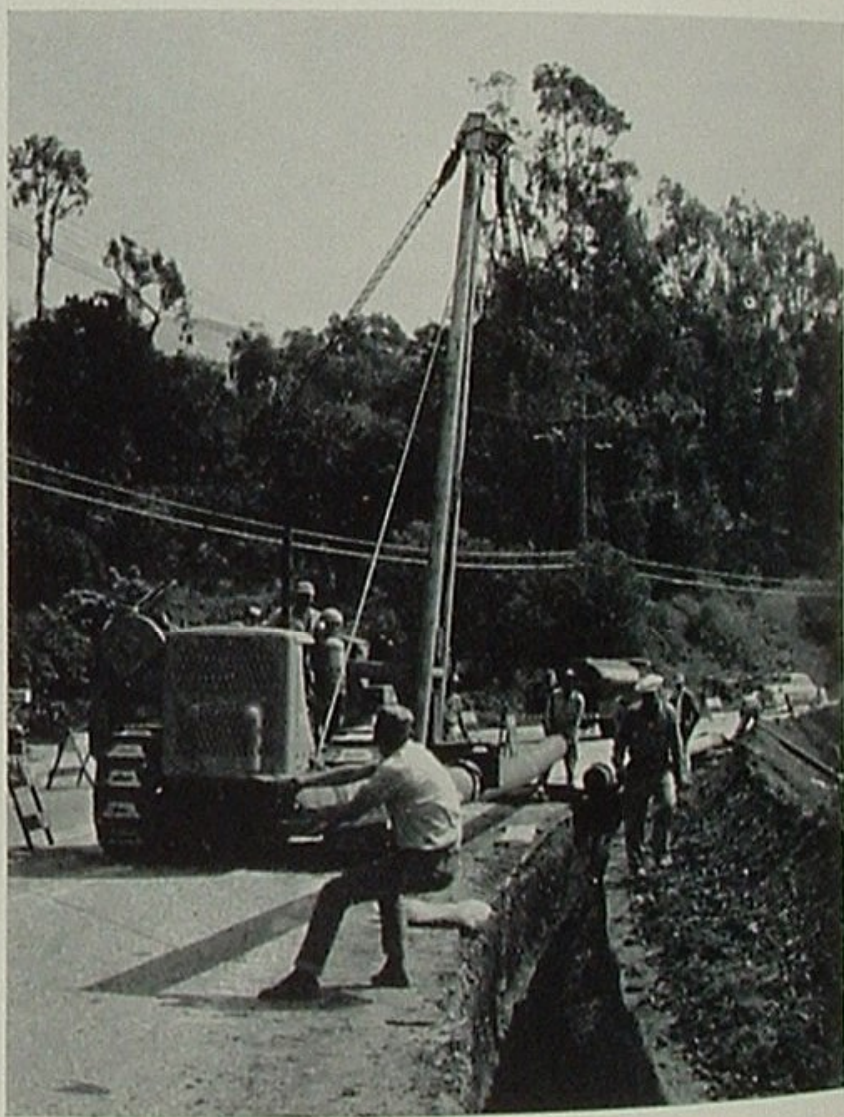
Construction of Torrey Pipeline was accomplished in six months by 150 men. Using petroleum-powered equipment, they dug 67 miles of trench through difficult terrain; transported, bent, welded, wrapped and placed an equal length of 12-inch pipe; and left only a surface indication of fresh earth or asphalt paving to mark the line's course.
