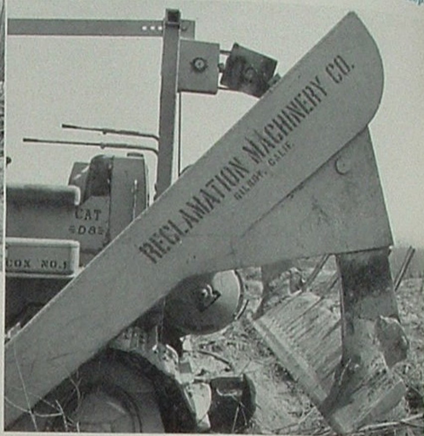
One of the diesel-powered tractors used effectively in Cibola Valley is equipped with a rake forward to bulldoze the covering of brush, and a self-sharpening knife (shown below in raised position) aft for shearing roots three feet deep.
