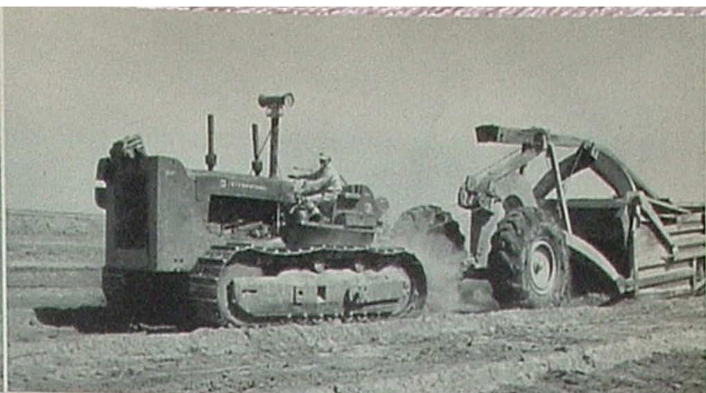
Large earthmovers invade the brush-cleared, fields to cut and fill uneven ground marked by rows of surveyors stakes.
