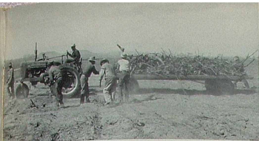
The only hand labor needed on this project is used to clear away roots and branches missed by the fire and rakes.
