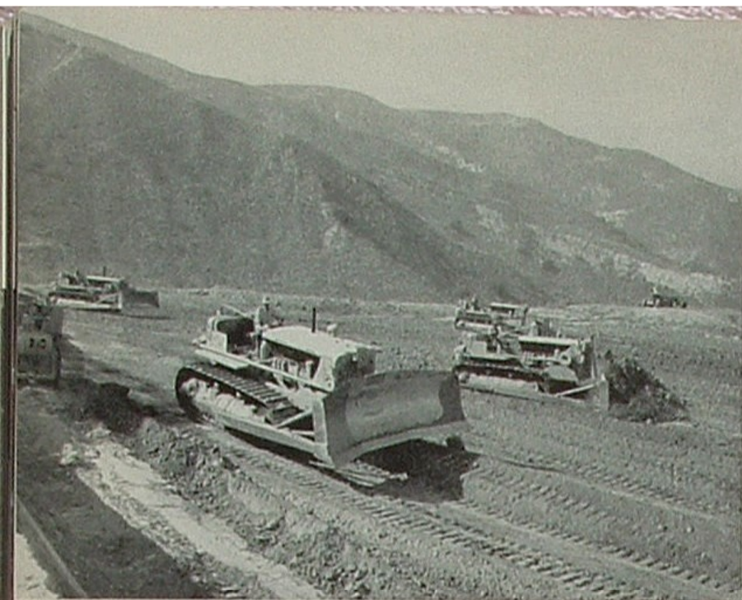
In our Santa Paula district, a mountain top is being bulldozed into Torrey Canyon, providing a level site for the construction of Torrey Pump Station. From here a new pipe line will be built to Los Angeles Refinery.
