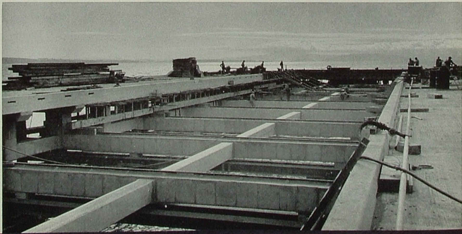
An immense new steel and concrete wharf is nearing completion at Oleum Refinery. It will accommodate four large
