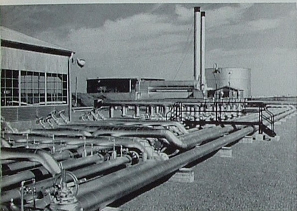
Oil pipe lines at the new station are installed above ground to facilitate identification of various systems.
