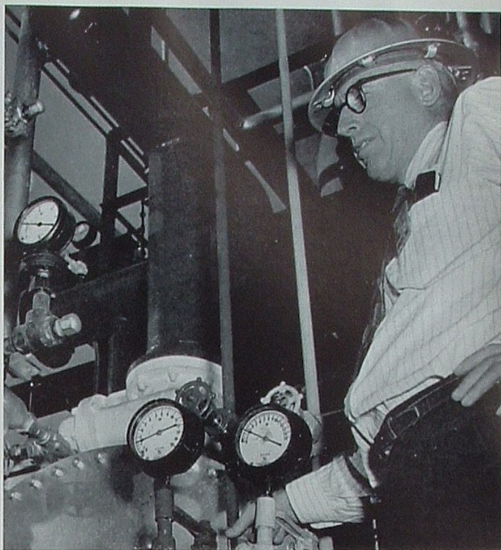
In charge of the new installation is Department Superintendent H. J. Jones, here inspecting main H 2 S furnace.
