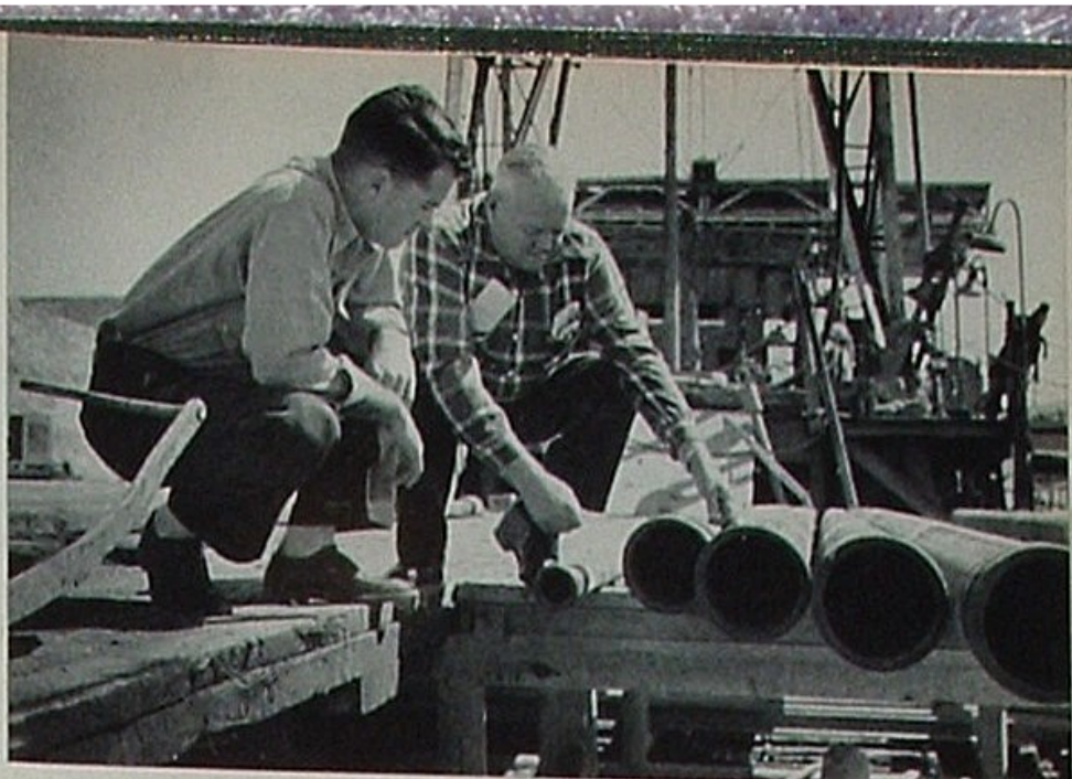
Hale Ingram, field engineer, and Charles Brown, drilling foreman, check diameter of casing that will line the well and of smaller tubing through which oil is produced.
