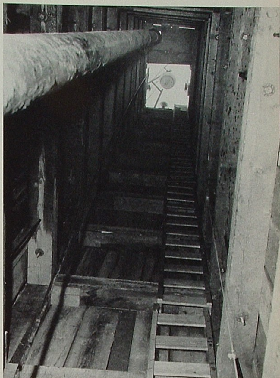
Looking upward from bottom of the 80-foot shaft, we see the reinstalled casing, top, and the protective space that will keep it from harm as the landslide continues.
