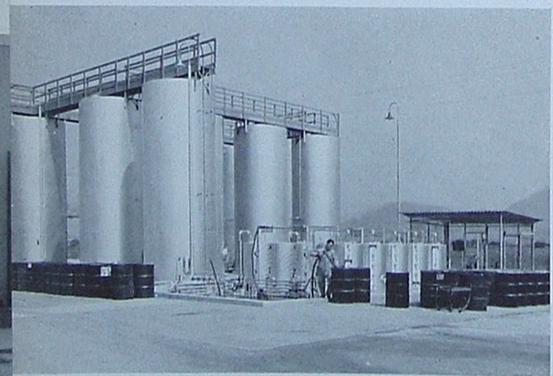
Two tank units, such as the one below, are used for fuel storage. There is also a covered barrel storage area.
