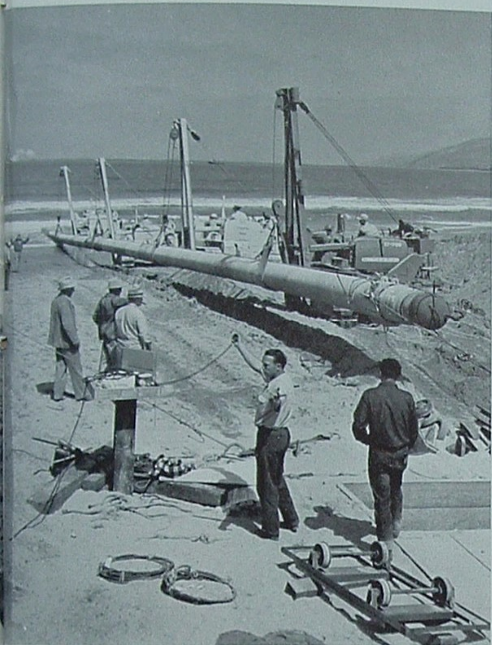
With the last section of 20-inch line being pulled and lifted into place, Howard Mollenkopf, Union Oil foreman, indicates by radio and gesture that a big job is done.
