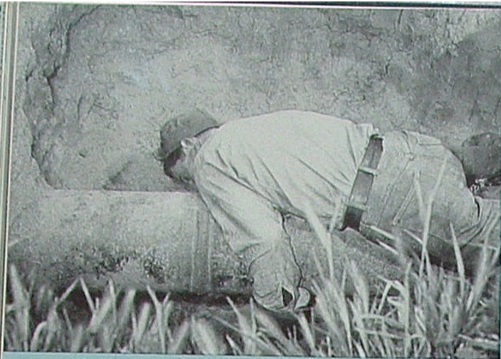
Looking for a leak of natural gas under a pipe line, Jim Head was suddenly overcome by gas that apparently filled the bottom of a four-foot excavation . . .
