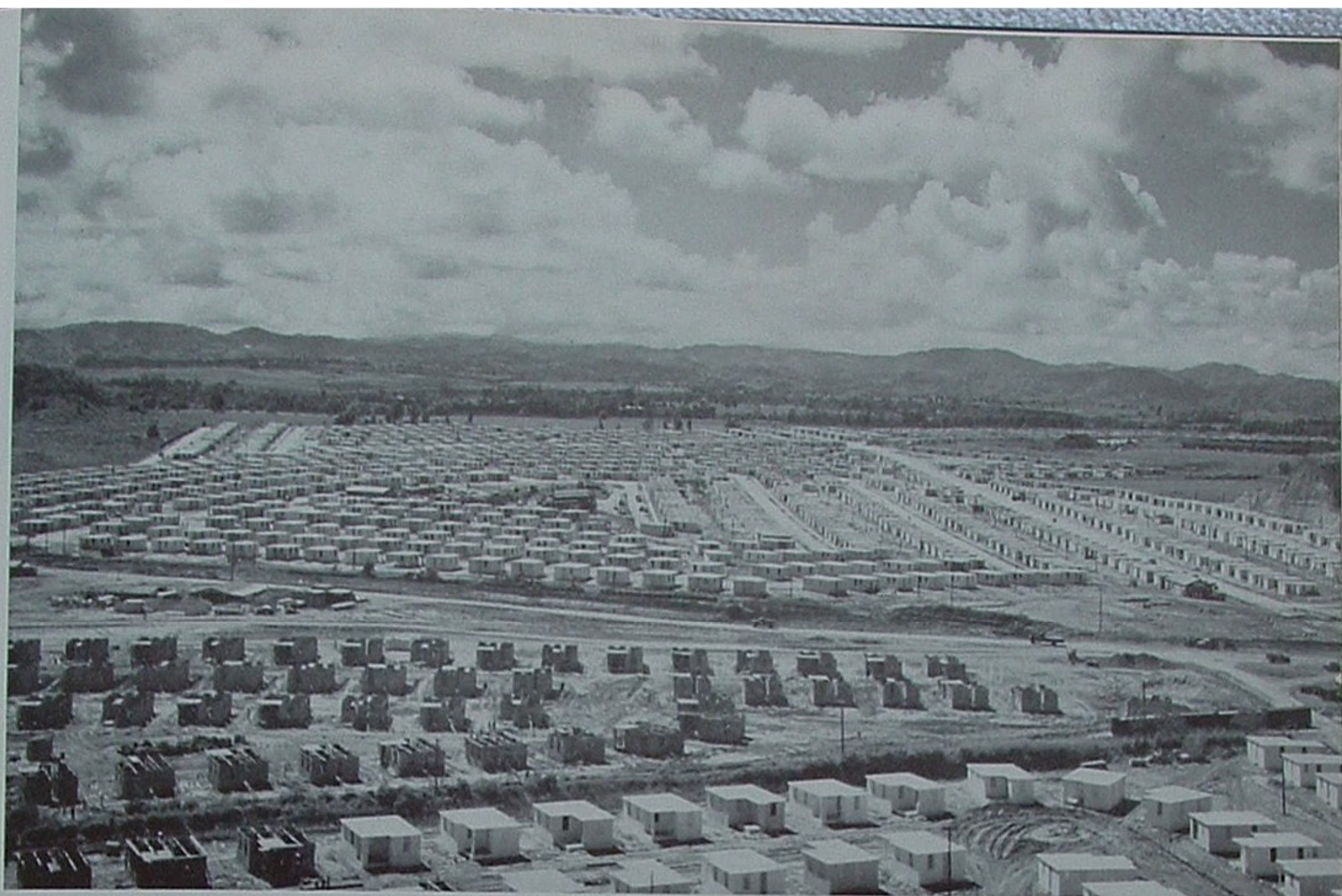
Here are some of 5,000 individual family units being constructed at Puerto Neuvo by Long Construction Co.
