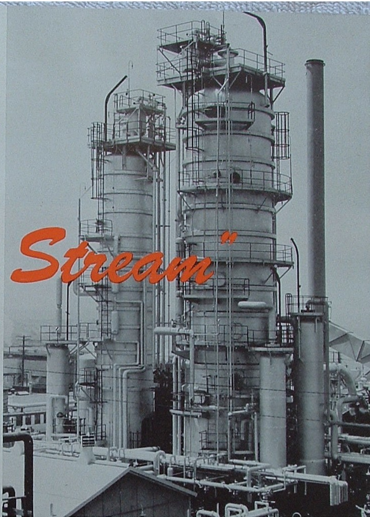
Unit 31 at Oleum includes the larger of these two vacuum columns, where Poso crude is distilled into gas oil, distillate and asphalt.
