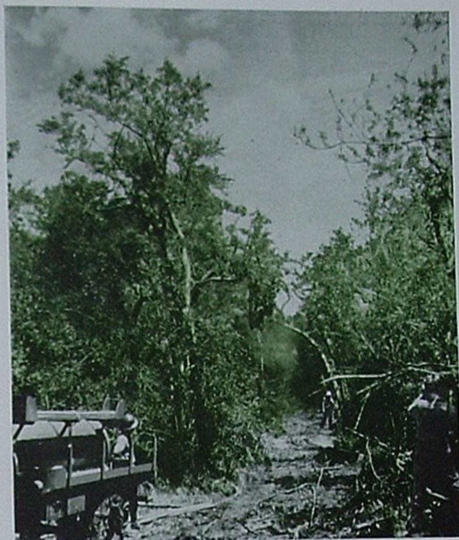
"As all work is carried on in the jungle, the tractors must go through first to clear a road of about cow-trail quality."
