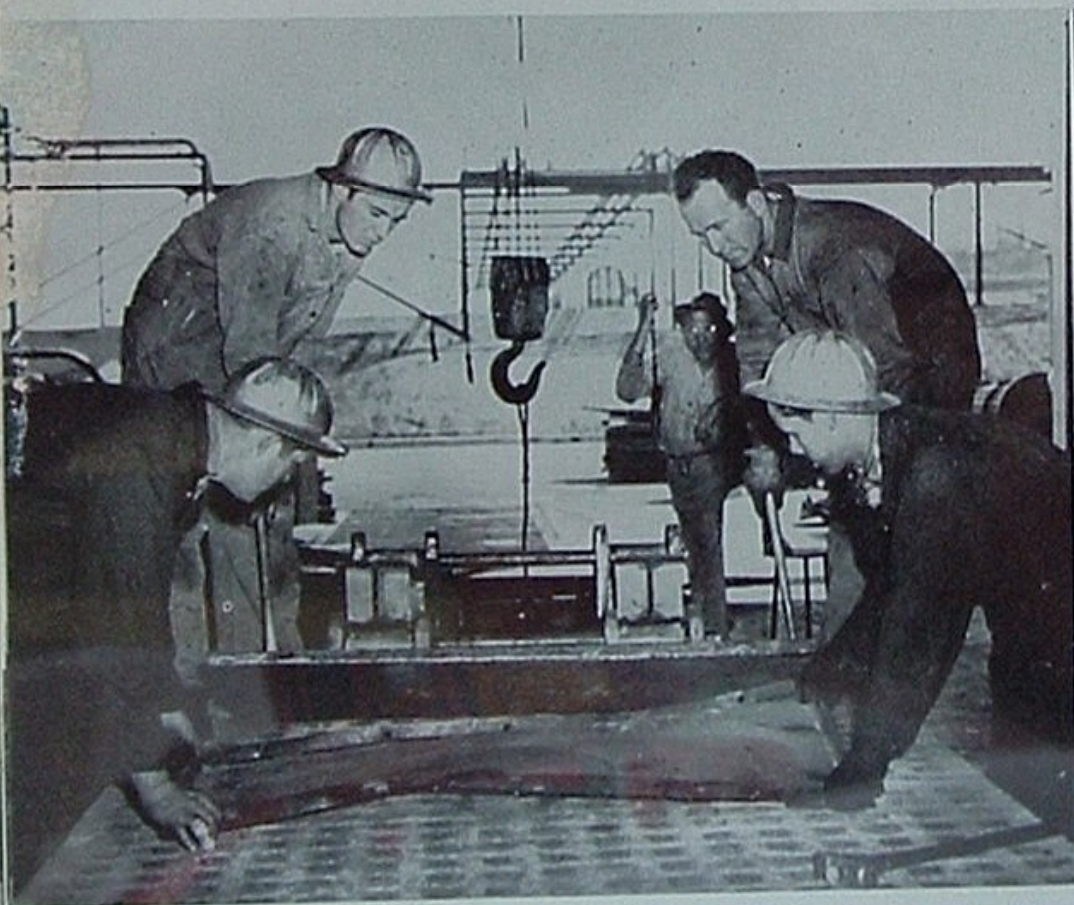
The refinery-designed press is capable of exerting an 80-ton pressure, more than sufficient to flatten the warped steel. Plate edges are pounded back into shape with sledgehammers.
