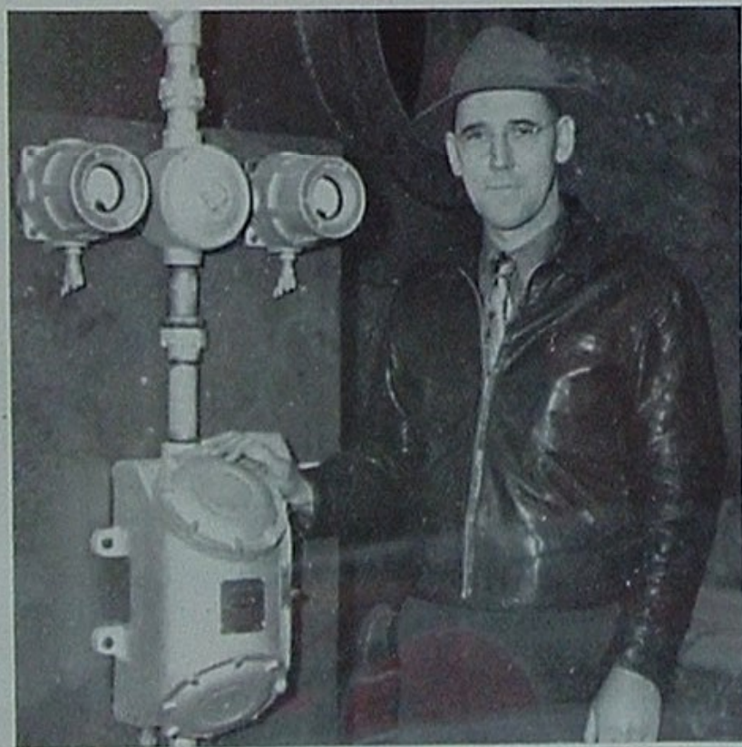
Associate Field Engineer Ira E. Triggs, author of this article, examines modernized control board of new electric dehydrator being installed at West Naranjal Lease, Brea.
