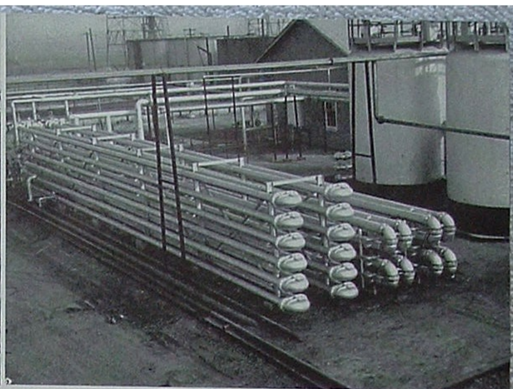
The two higher banks of pipe at left are heat interchangers, wherein out-going dry oil imparts some of its heat to the incoming wet oil. Steam interchangers, pipes at right, complete heating process.
