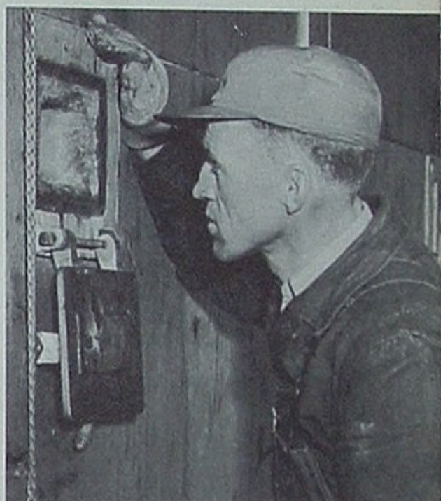
Believe it or not, the burners in this refinery furnace froze up during the below zero weather. Operator is Fred Webster.
