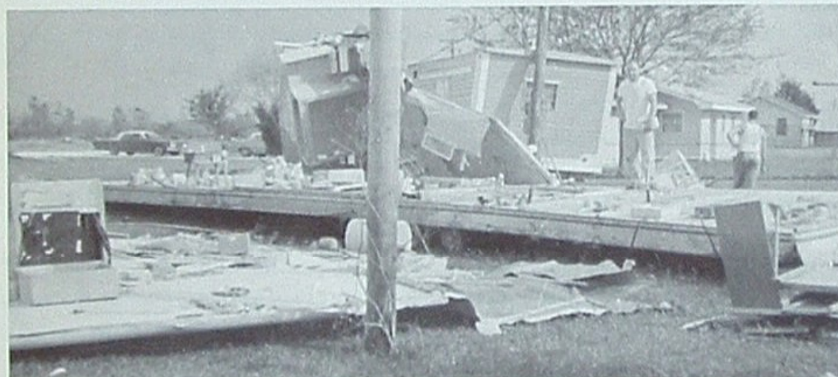
This demolished trailer house was the remains of Naquin home after Hurricane Betsy.
