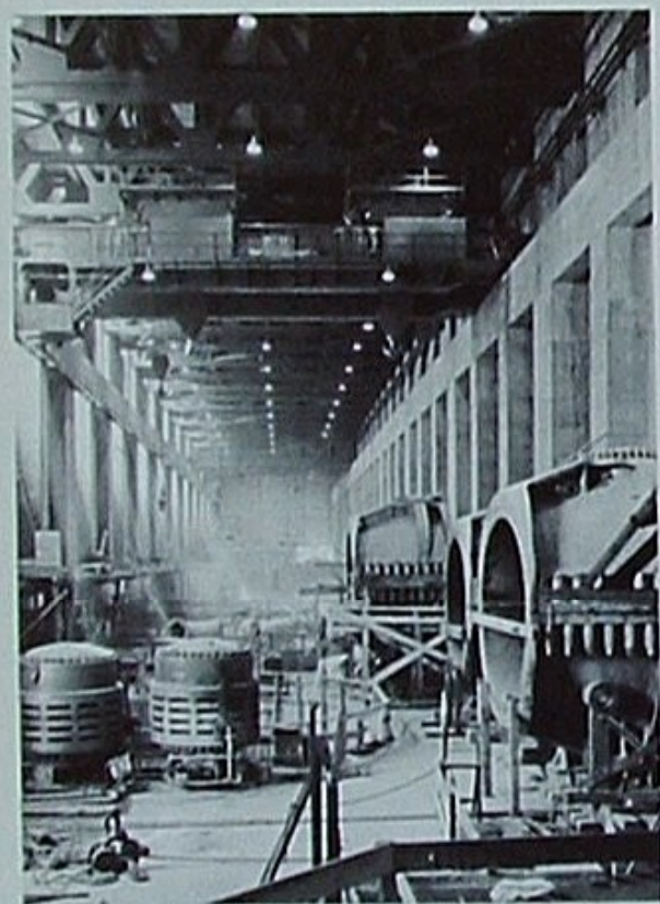
Los Angeles got its first electrical power from the dam in 1936.
