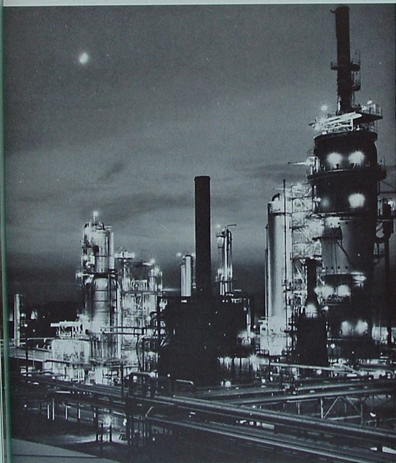
Orthoflow fluid cracking unit at Smith's Bluff Refinery, Nederland, Texas.
