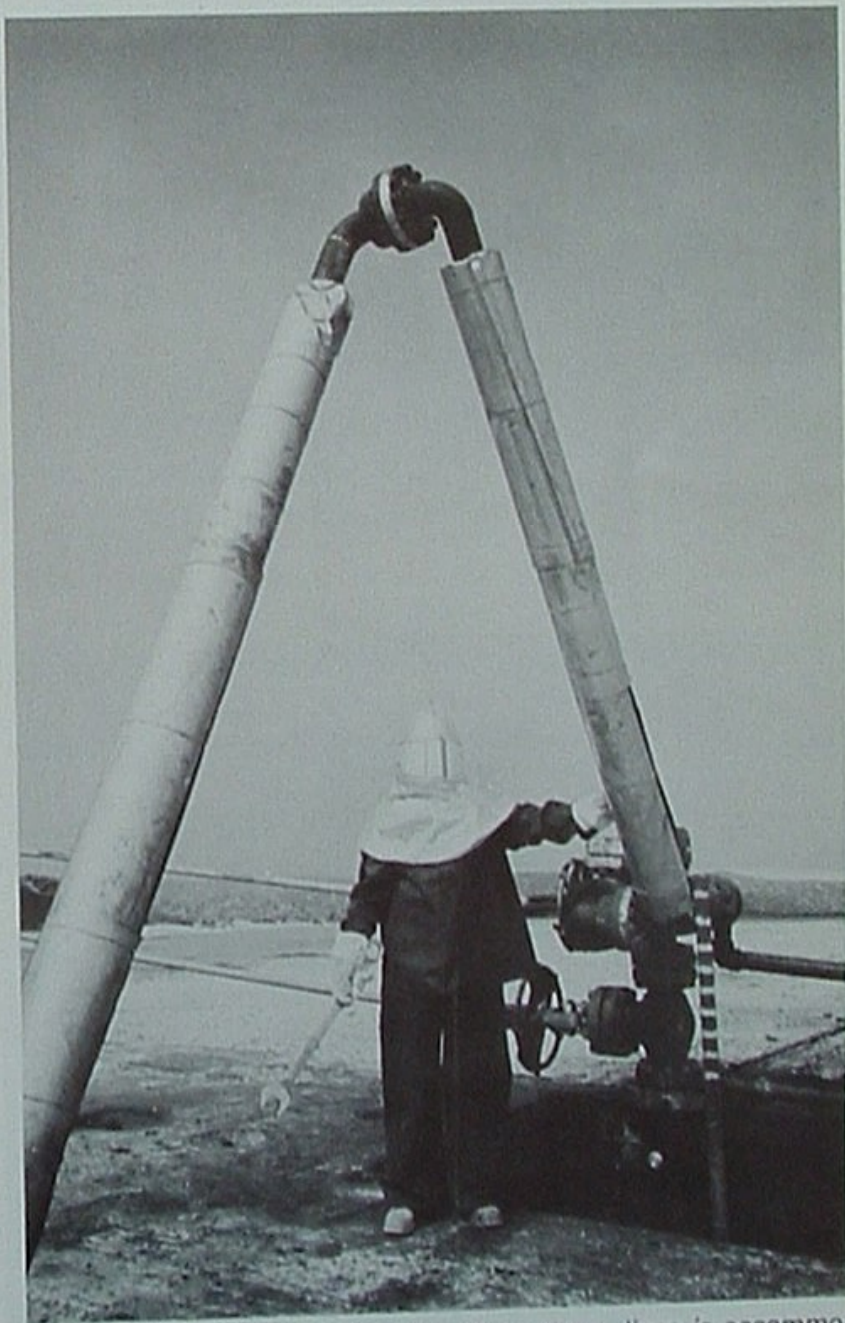
STEAM RETURNS: Expansion of surface steam lines is accommodated by swing joints. Lines exposed on surface are insulated.
