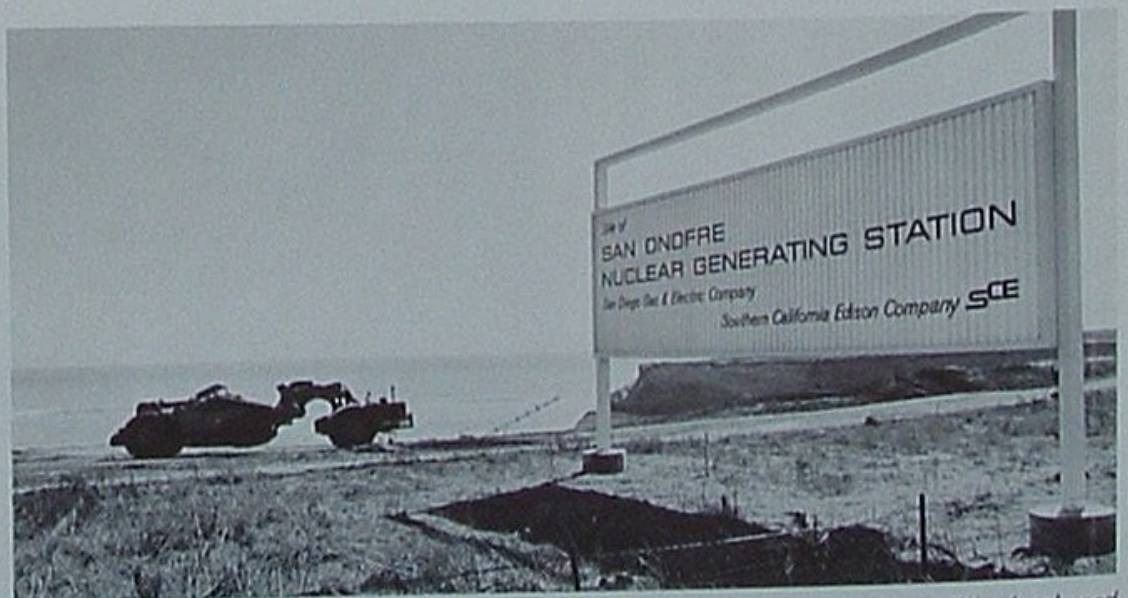
NUCLEAR GENERATOR: Earthmoving machines, each hauling enough to fill a backyard swimming pool, were powered by Union fuels during site preparation for plant.
