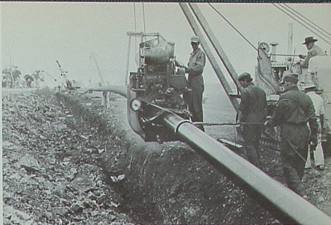
Before oil could be marketed, Union and partners built a 10-inch pipeline to Lytton, near Brisbane. Bechtel was builder.
