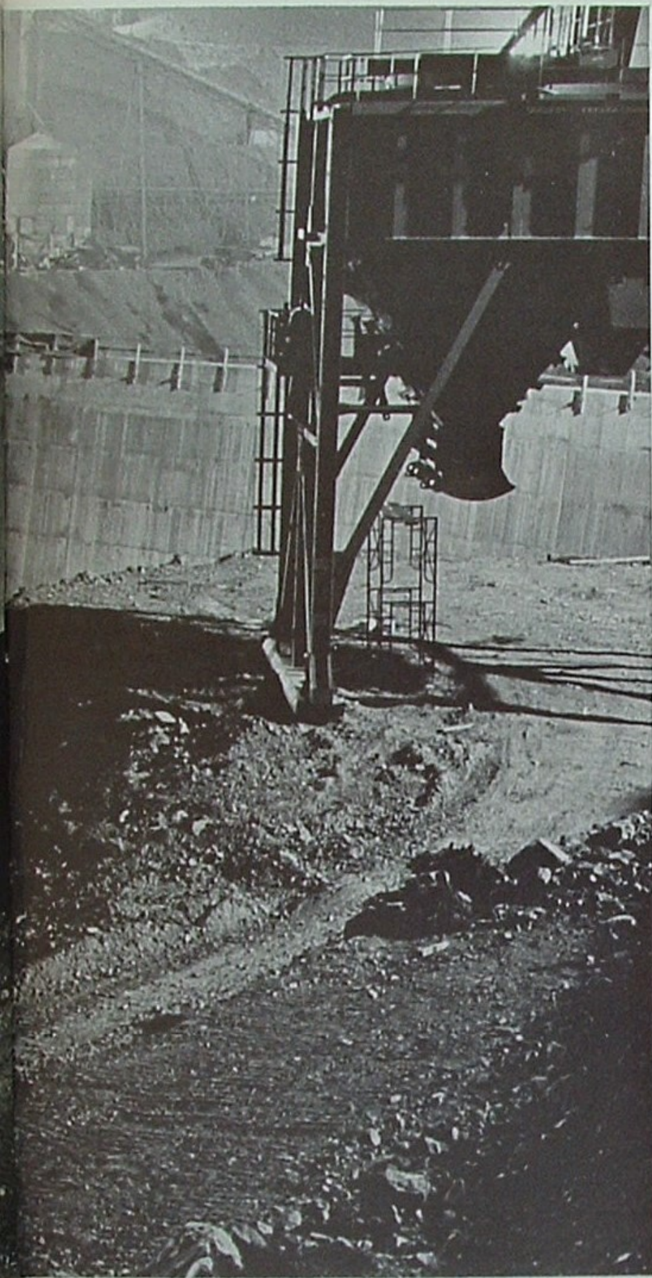
Working day and night, Oro Dam Constructors first poured an immense concrete core to block the Feather River. The earth-fill dam rising high above the core will begin history's biggest water project.
