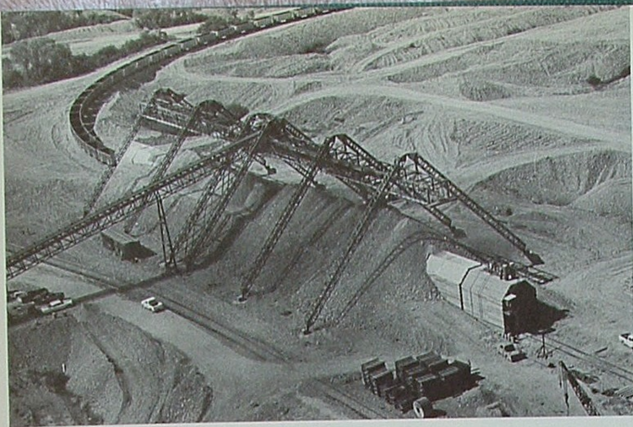
Materials for the earth fill are obtained from old gold-dredging deposits near Oroville. Under the railway stockpile, supplied by conveyor belts, a 40-car train can be loaded in about 14 minutes.
