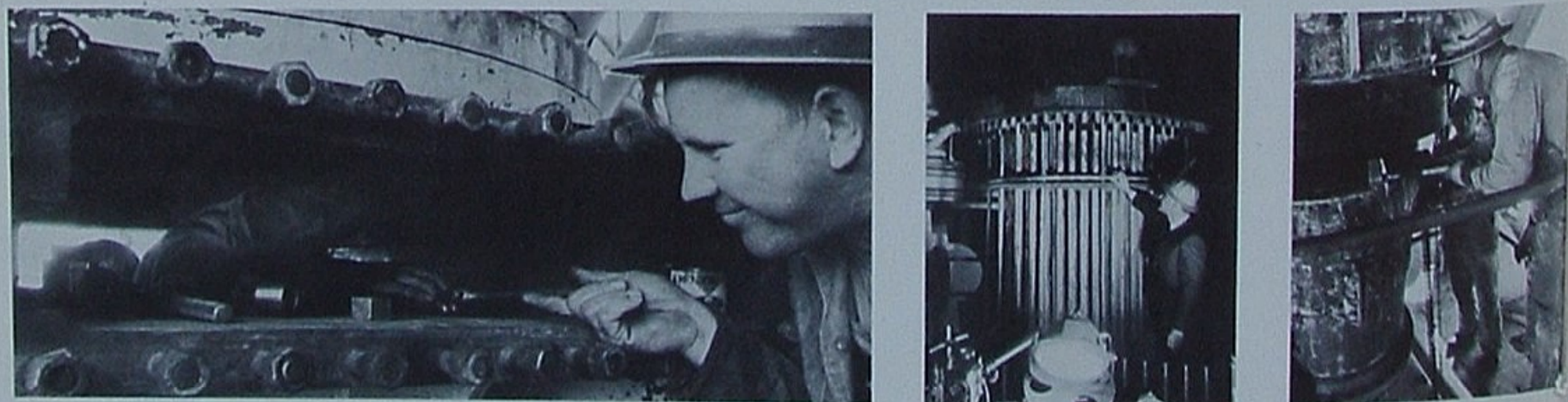
Above: Machinist Riley Baker is inside that big slide valve; Walter Goron is handing him the wrench. Center: Supervisor of Planning Ward Stennett checks the status of repair work on the Fluid Cracker's steam generators. Right: Inspector Wylie Day, in background, watches as contractor employee loosens bolts in flange.
