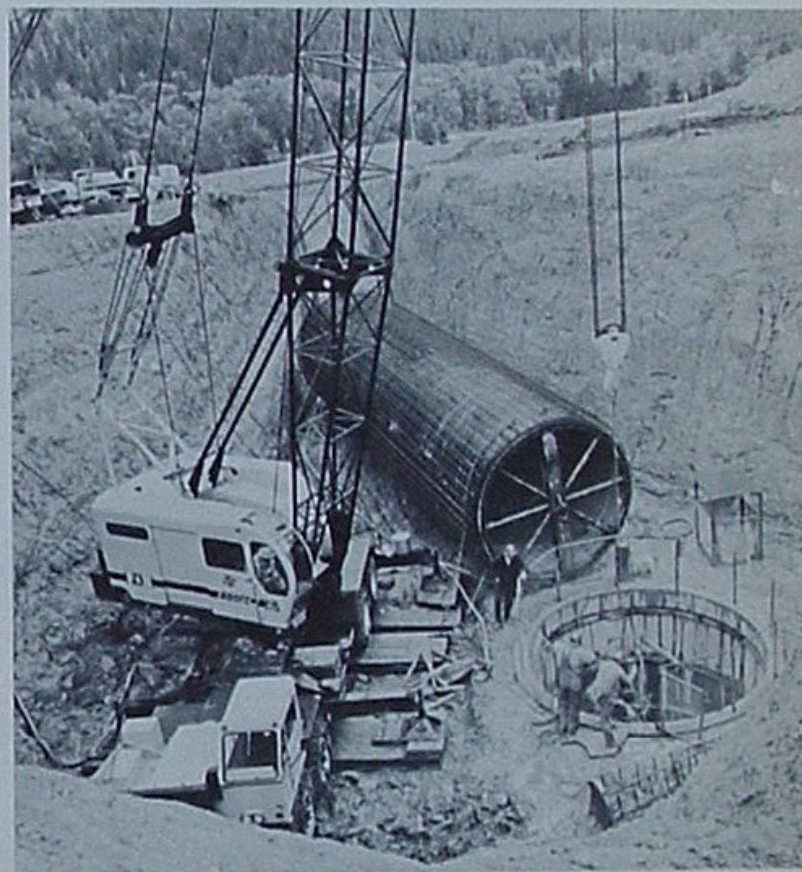
25-ton steel liner ready to be lowered into a Minuteman silo on the Montana plains.
