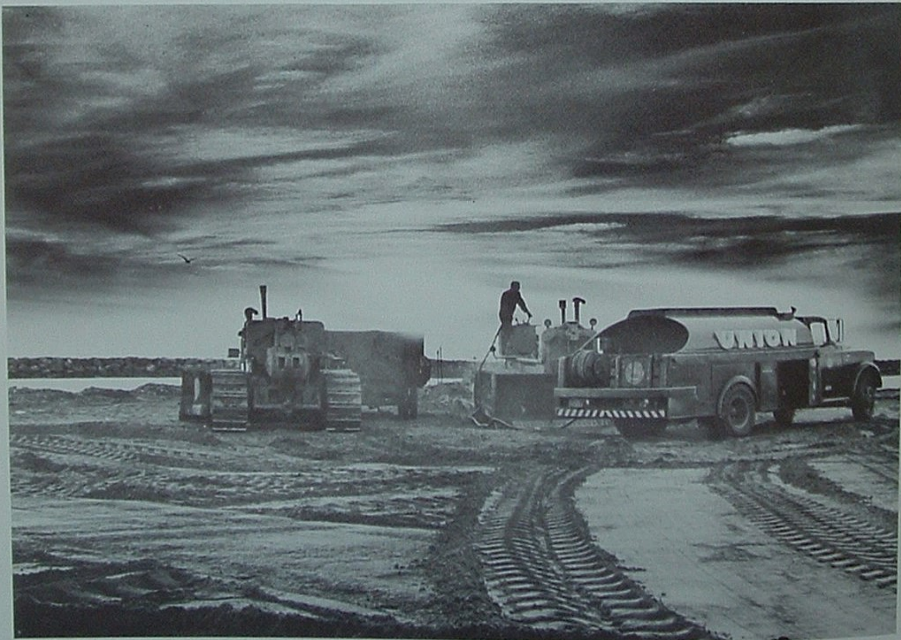
Union Oil service truck refueling some equipment at site of Redondo Beach King Harbor Development.
