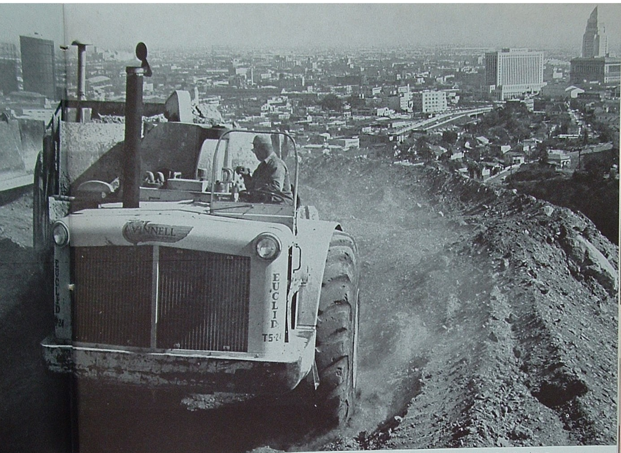
High above downtown Los Angeles, a mighty earthmover powered with 76 Unifuel sweeps around a curve during the construction of the Dodgers' ballpark in Chavez Ravine. Contractor: Vinnell Constructors.
