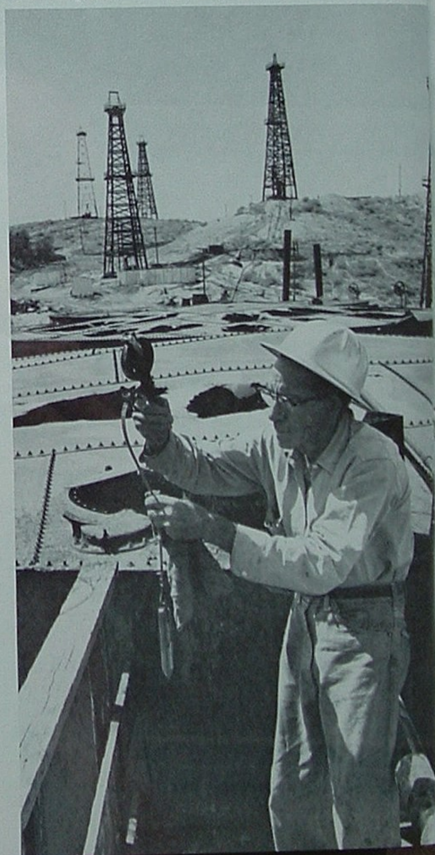
Holes eaten in tank tops by sulfur fumes are no reflection on the field operator — the field simply doesn't earn repairs.
