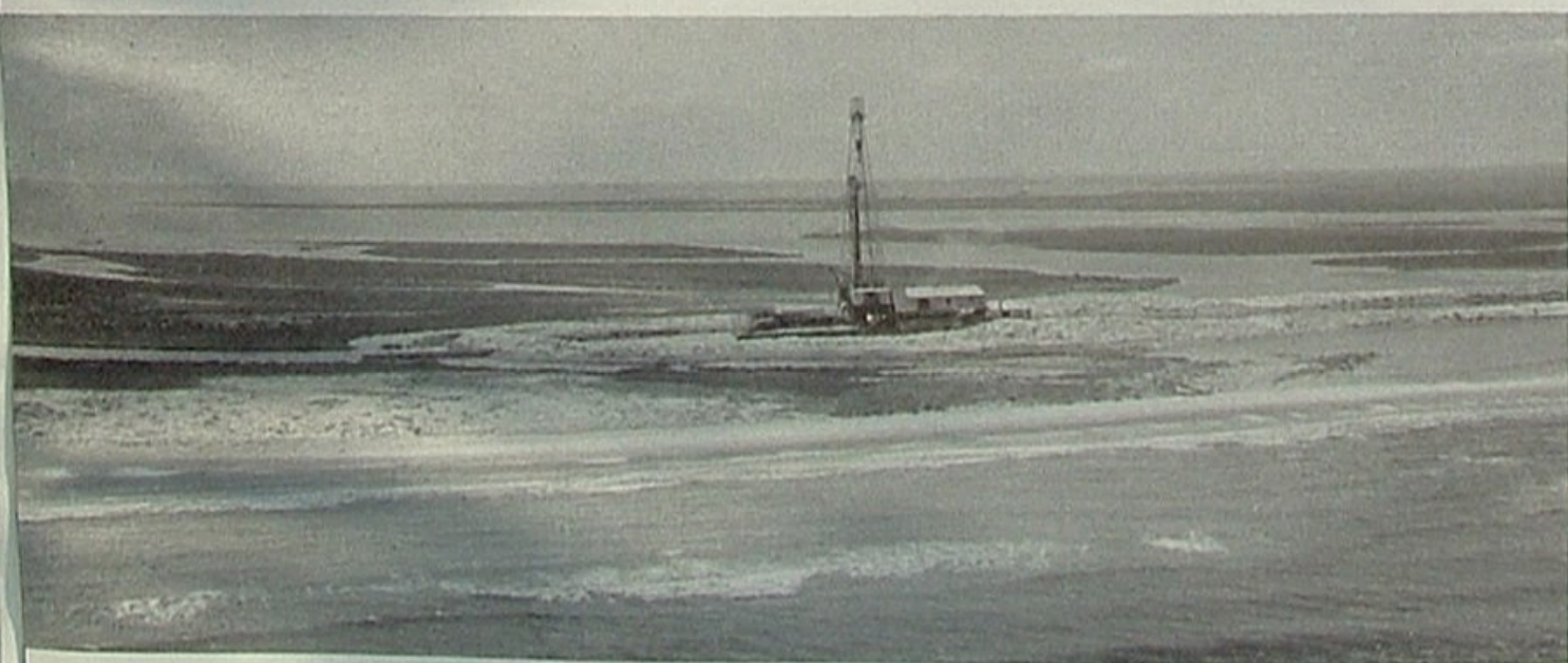
But human skill and persistence finished the job. Here on a narrow strip of mud between Timbalier Bay and waves of the Gulf of Mexico is the start of another oil field—Union Oil's deepest drilling effort—fourth deepest producer in the world.
