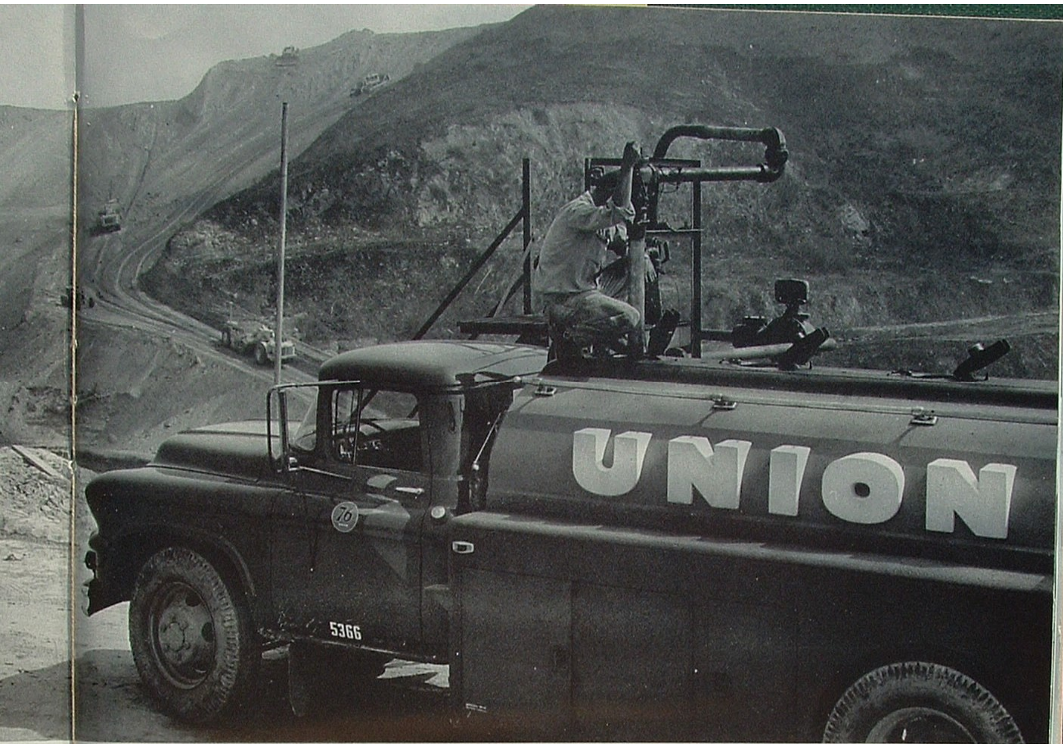
"Batteries for today's game" in Chavez Ravine are a 76 pump "on the mound" and a tanktruck "receiving." In area being leveled by earthmovers, over 50,000 fans soon will root for Dodgers.
