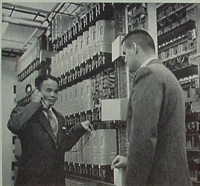
NGUYEN LUYEN, left, a radio technician from Vietnam, is studying American communications as a guest of the Federal Communications Commission. He regarded Union Oil's microwave system at the Center as an outstanding feature of his schooling. Tutoring the Vietnamese during his Union Oil sojourn was Trainee Ron Kunzelman, who is studying toward an engineering degree at California Institute of Technology.
