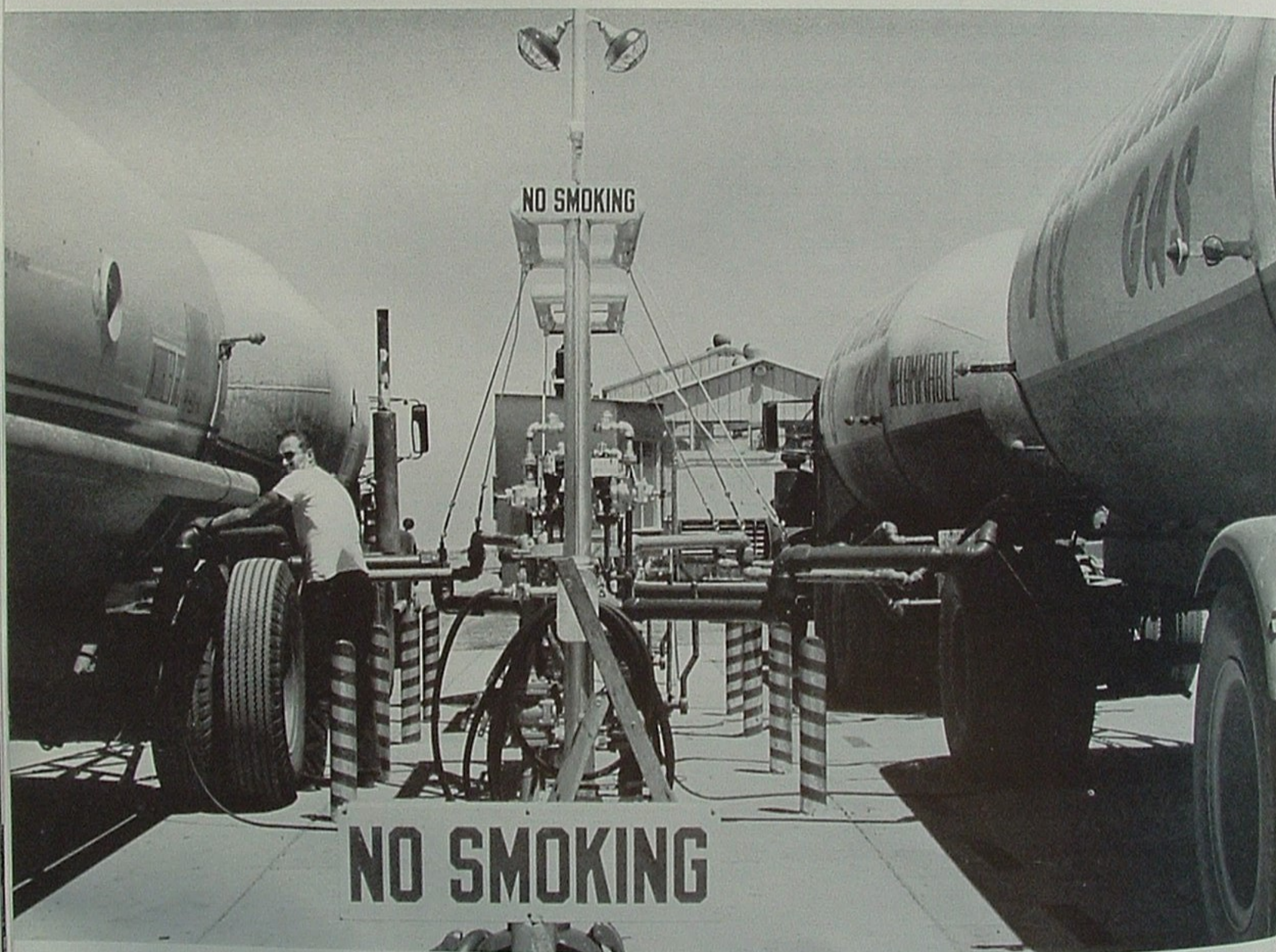
Operator Steve Hoag at Polvadero Field is reversing the usual process; he's receiving two loads of LPG for delivery to the oil field.
