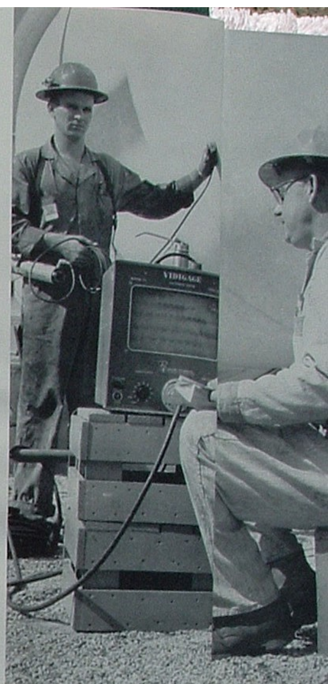
The Vidigage here being used on an LPG tank by Kellogg and Wylie Day measures wall thickness by sound-wave technique.
