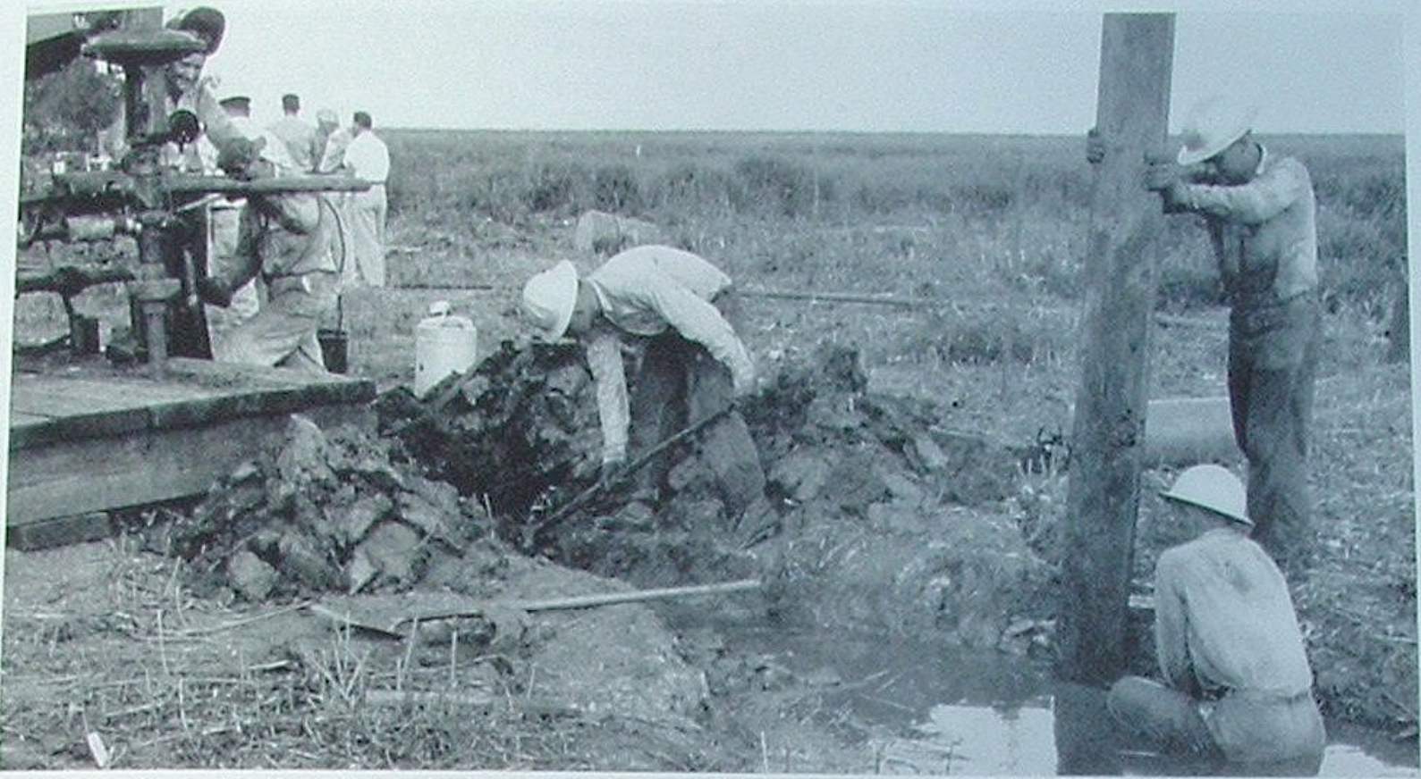
Repairing a gas pipeline near Houma, workmen contend with the water table, which in the marsh adjoining the Gulf of Mexico is seldom more than a foot underground. Pipe corrosion is a serious problem in gas fields.
