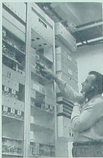
John Reed is one of 16 repairmen who keep system in good order.
