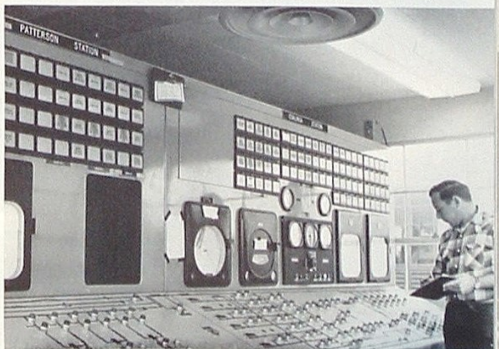
Senior Engineer Mel Whiteday, on one-man operating shift at Coalinga, also controls Patterson through microwave contact.
