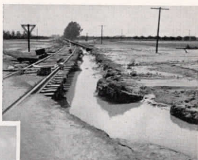
Above: Santa Fe railway tracks to San Diego. Note how water has undermined the ties.
