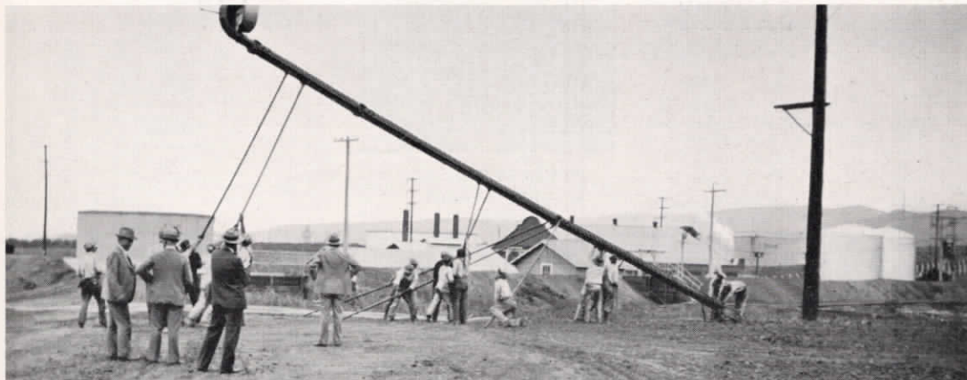
Fire drill at Stewart pump station, Los Angeles pipe line, showing erection of a portable foam tower.
