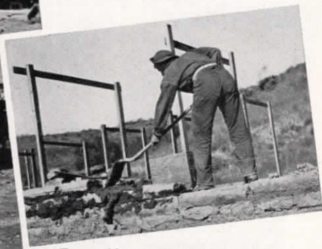
Above: Spreading adobe mortar with a shovel may not be scientific, but it's effective.
