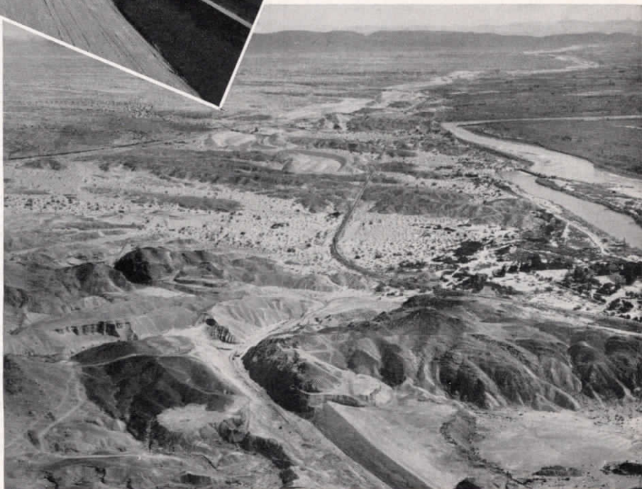
Above: A completed portion of the canal. The small dot in the center is a workman, which will give some impression of the size of the project.
