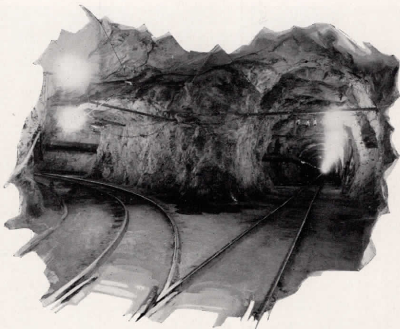
Adit "Y" junction with main tunnel in the Whipple Mountain tunnel under construction by Walsh Construction Company. Completed tunnel will be 10 miles long.
